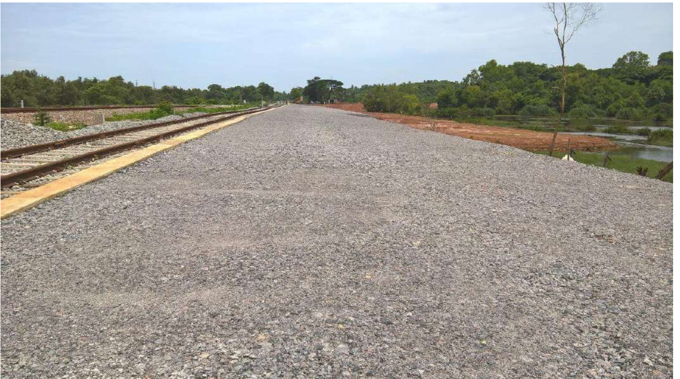
Creation of New Assets – Half-rake length Siding at Thokur Yard near Mangalore, Karnataka
